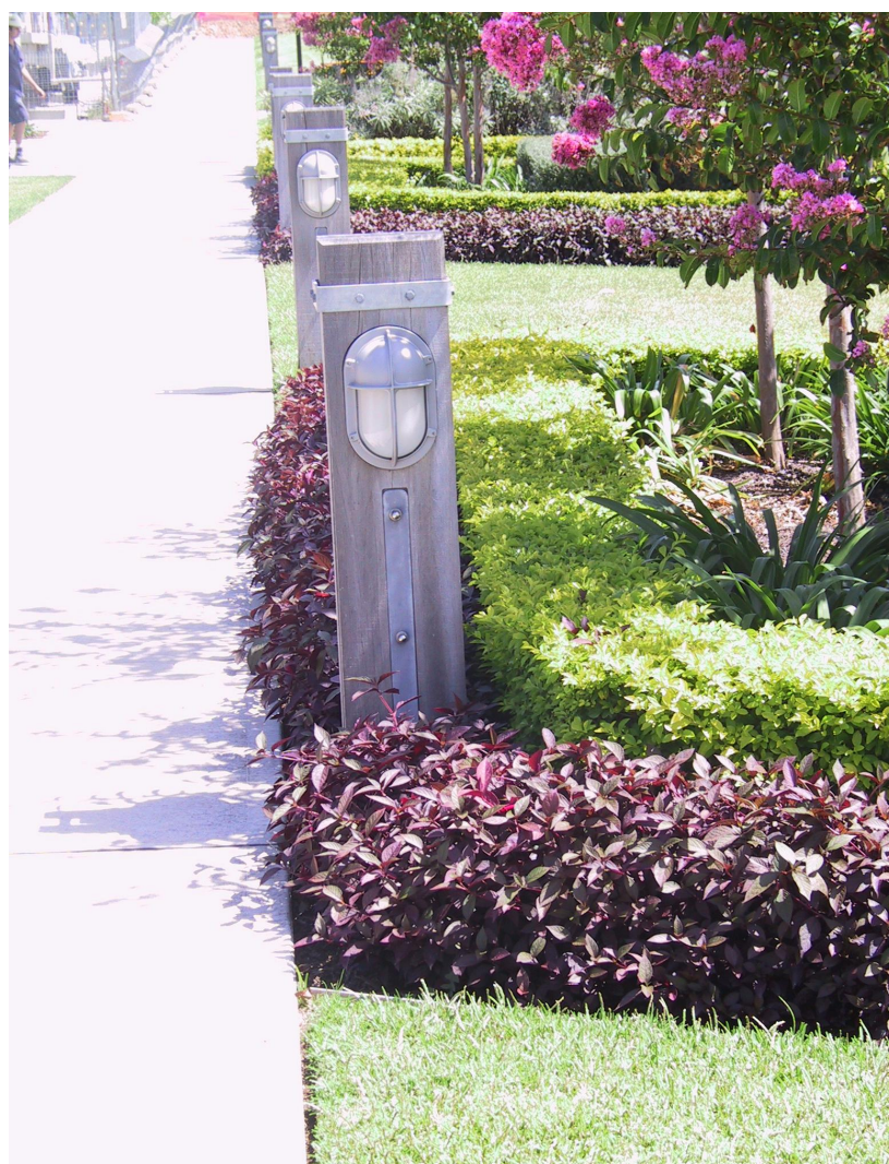
Low level bollard lighting
